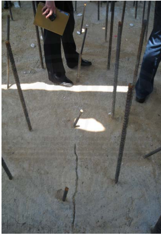
Fig. 8.39 Crack on top surface of a footing
