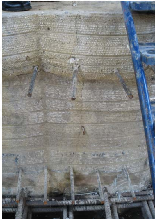
Fig. 8.40 Crack on side surface of a footing
